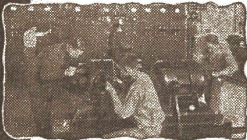
Students repairing motor generator set, and operating one of our power switchboards.
